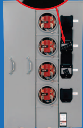
4 gang 200A per position All-In-One Meter with all covers installed
