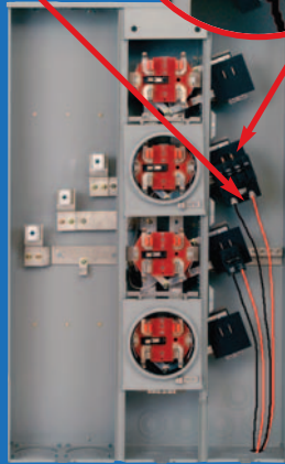
4 gang 200A per position All-In-One Meter with 100A and 200A circuit breakers installed
