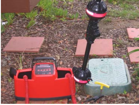
Figure 8: Checking the Signal
